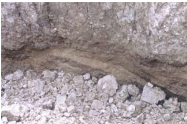
Figure 3. Cave-In Area (Looking South, cave-in area is approximately 30 feet long and 11 to 13 feet deep.)
