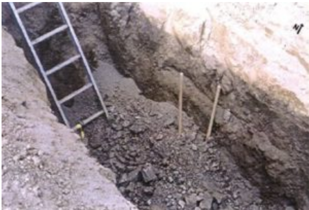
Figure 4. Incident Scene (The victim and his co-worker were buried near the west end of the trench.)
